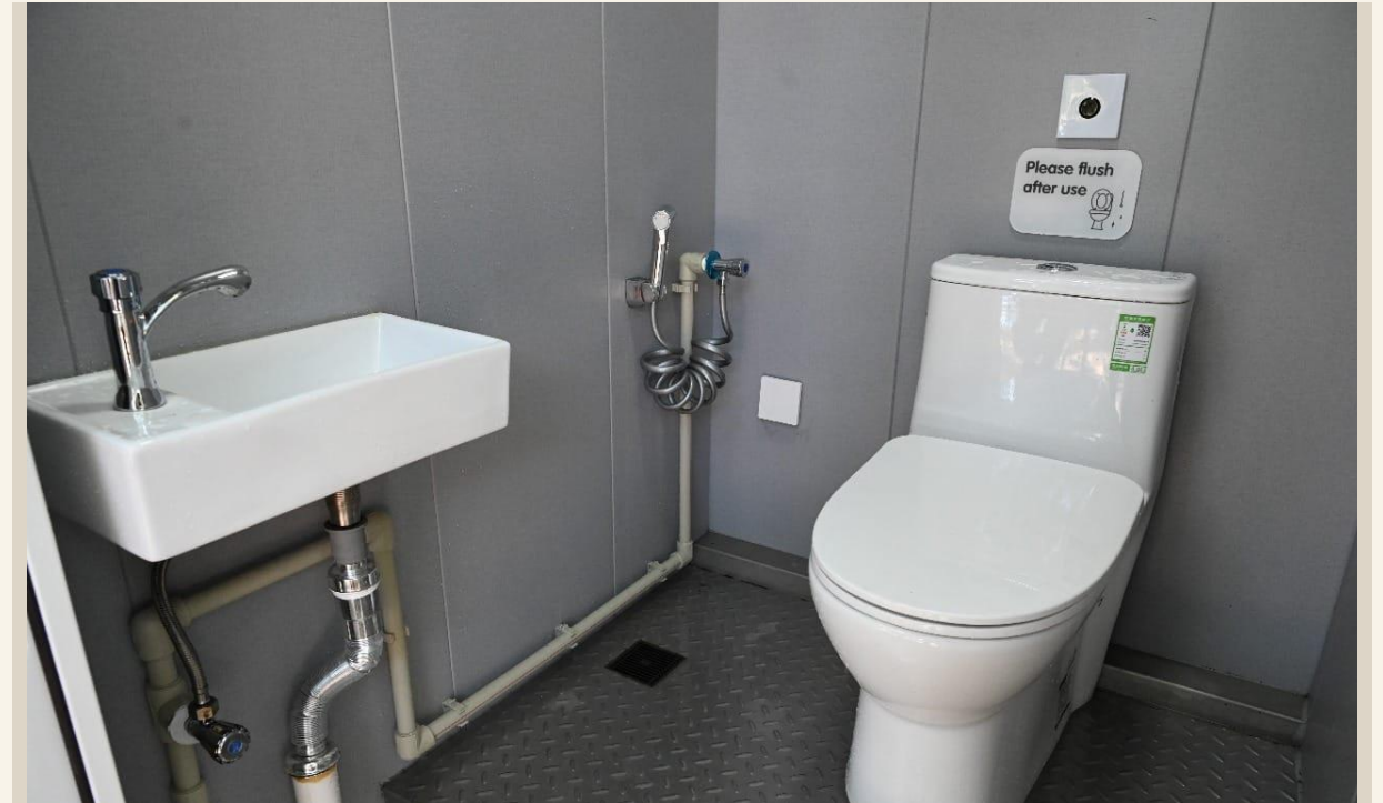
Lumbini Park · WC, washbasin and hand spray
