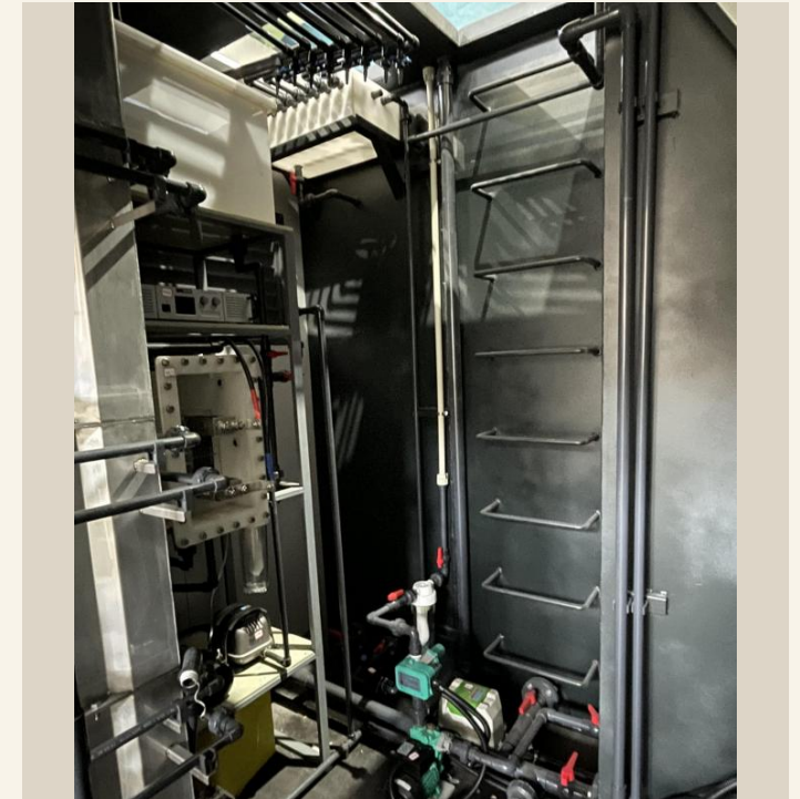
Factory view · Treatment equipment and pipework
