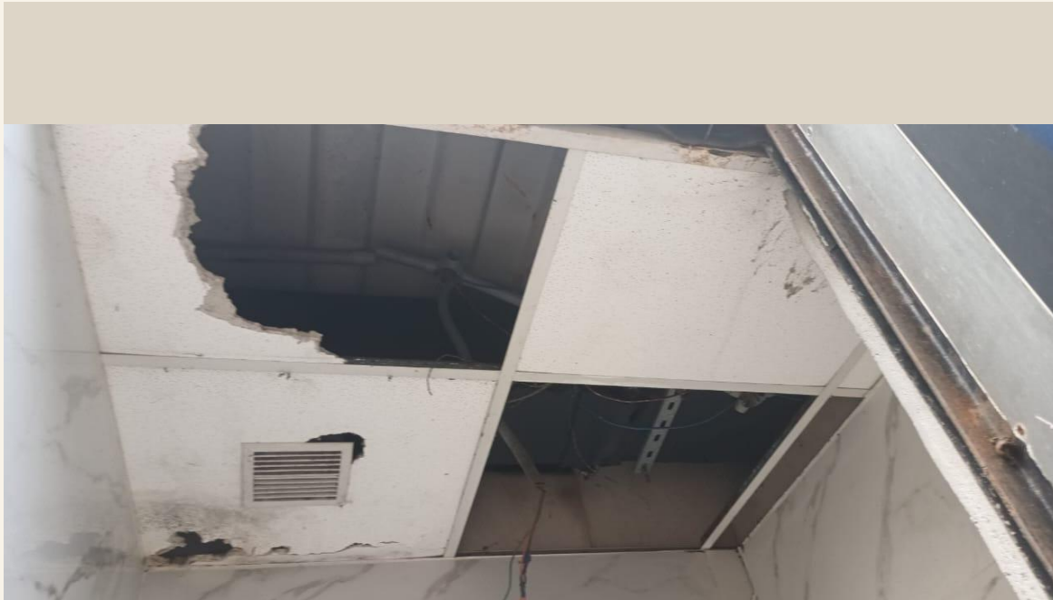
Damaged ceiling · Before section, 9 September 2024
