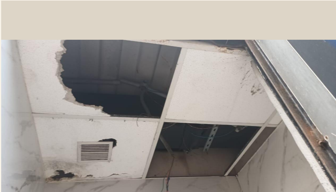
Damaged ceiling · Before section, 9 September 2024
